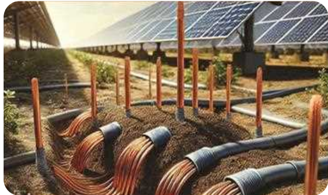
EARTHING & GROUNDING FOR PV PLANT . PIC Courtesy @ PRASUN BARUA
