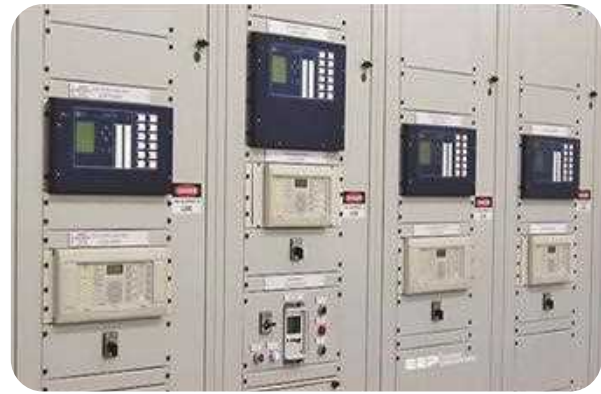
PROTECTIVE RELAYS PIC COURTESY @CLEANTEC CONTROLS1
